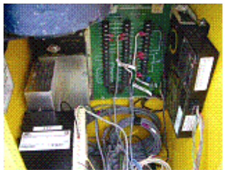
A new controller from Magnetics and a network connection were placed in the gate.
